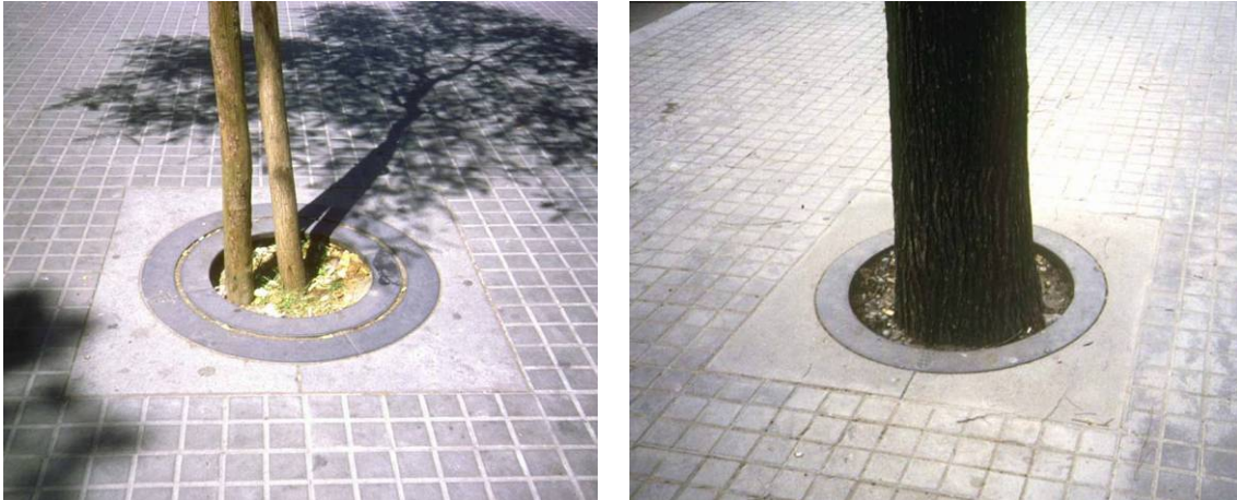
Fig.5 and 6. Another complex problem is to solve the limits between a pavement and a space around tree trunks. The examples of tree grates shown above allow the correct growth of the tree; concrete slabs that limit the tree well are easy to adapt to a walkway pavement and concentric cast-iron rings are resistant and non-deformable.
